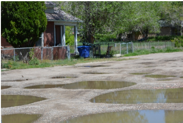
Southwest view of the road condition
